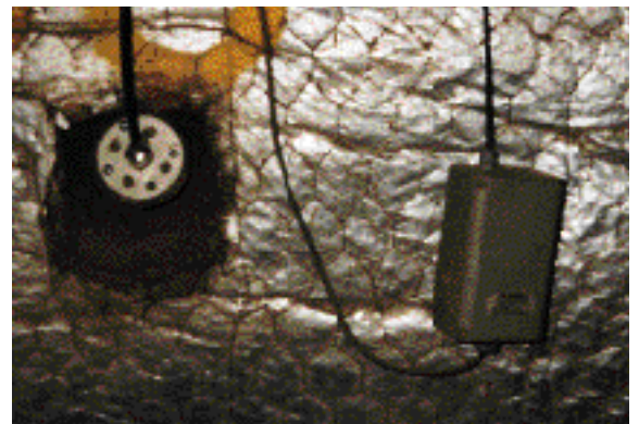
A Vaisala humidity and temperature transmitter in the dryer recirculation system.
